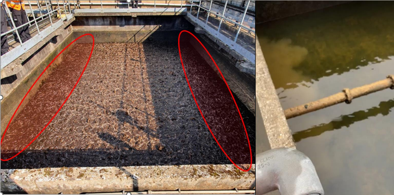
FIGURE 16: FONTBURN RGF – DEADSPOTS DURING BACKWASH
